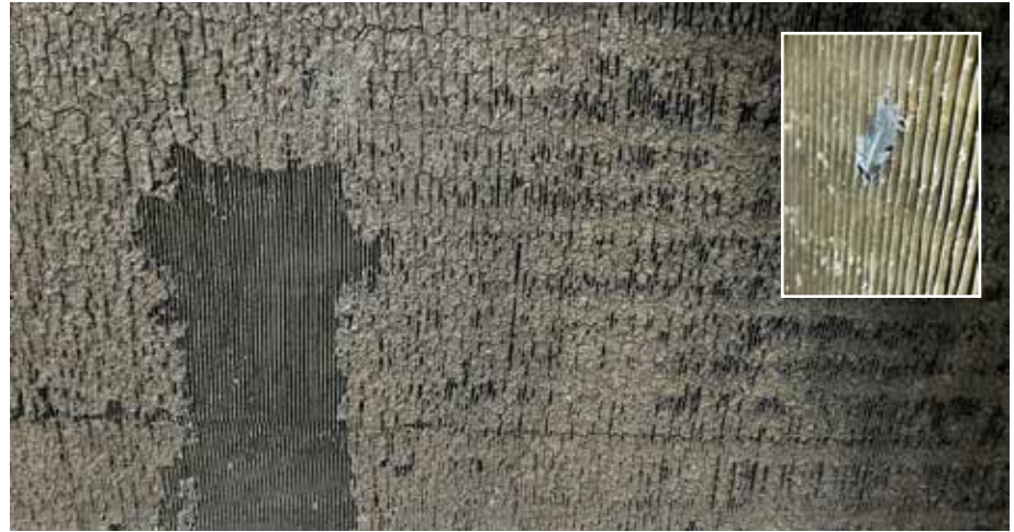
Figure 1: Dust-cake formation buildup on a cooling coil (top-right: Pigeon’s feather trapped on cooling coil)
