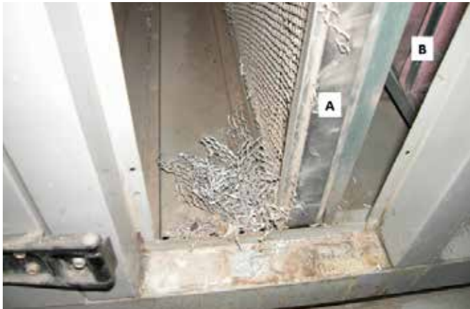
A typical filtration stage illustrates corroded low-efficiency pre-filters [A] and conventional pocket filters [B] installed in air-handling units
