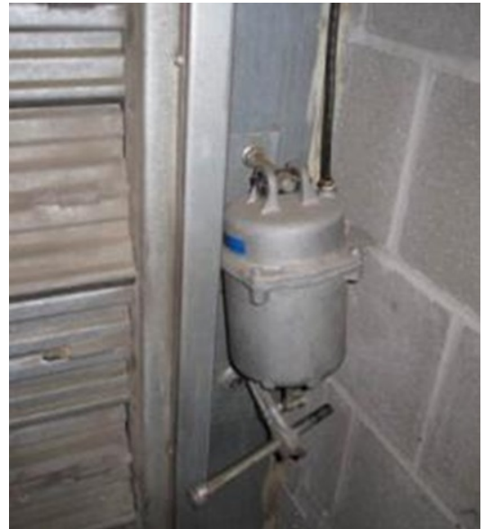
Outdoor Air Actuator: Disconnected, thus no outdoor air is provided for building occupants (unintentional reduction of OA)
