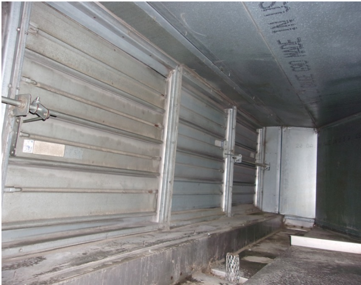
Outdoor Air Damper shut: This damper is intentionally shut, thus ensuring no OA for building occupants
